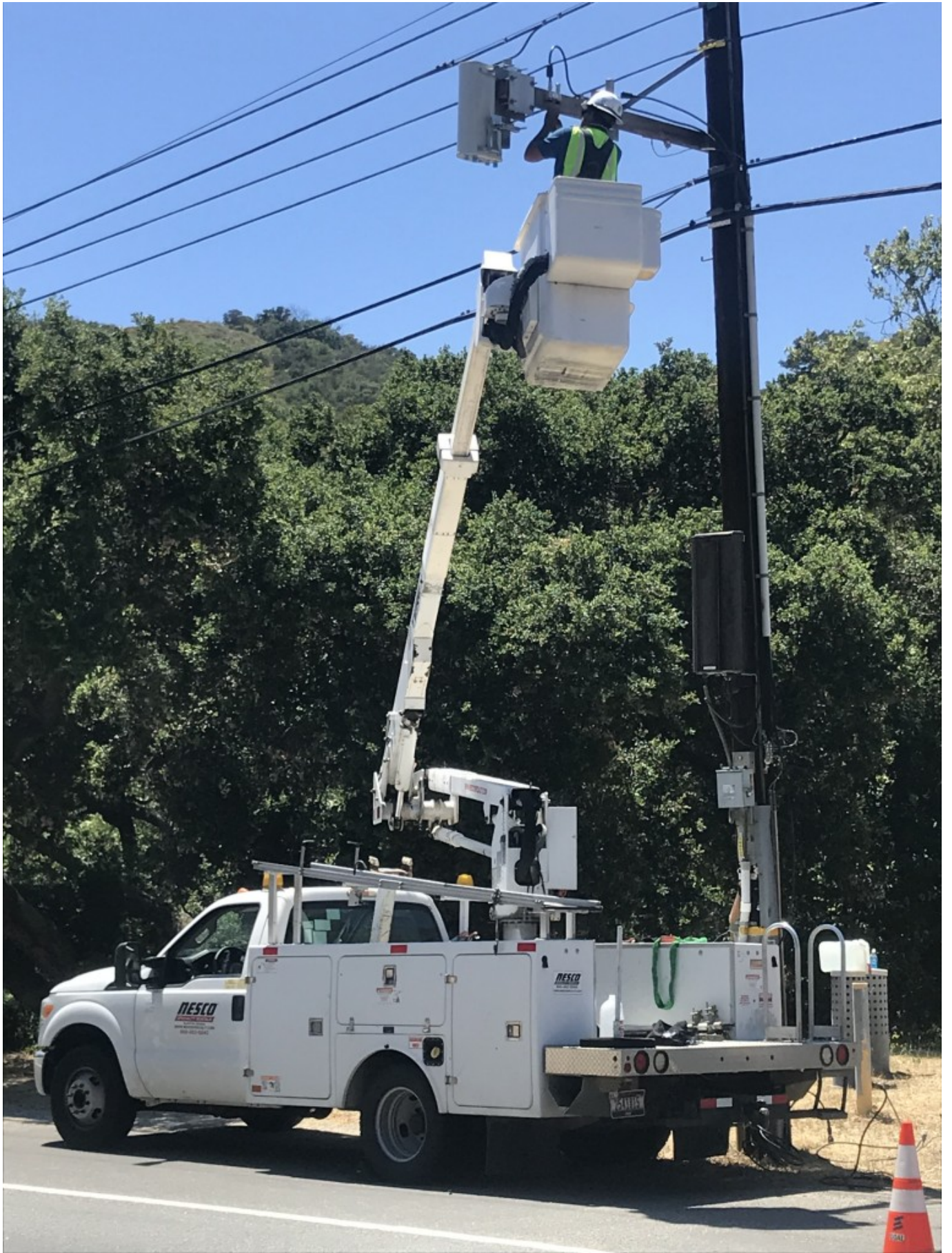
An aware public in the key to backing off the barrage of illegal installations.
